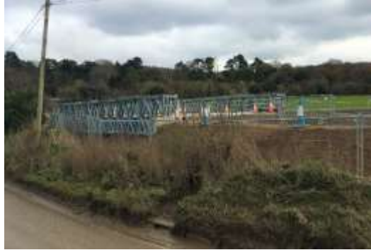
HS2 are constructing a ventilation vent in this valley. This bridge takes construction vehicles over the river.
